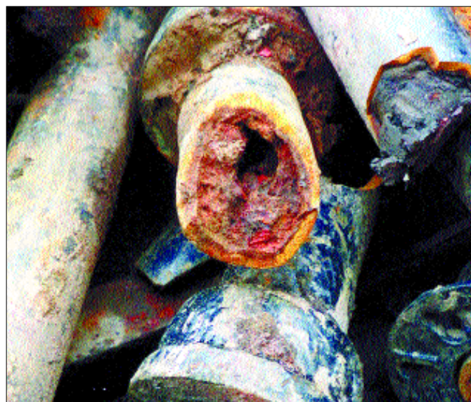
An example of the condition of the old pipes that are being replaced on the Jaguariuna pipeline project.
