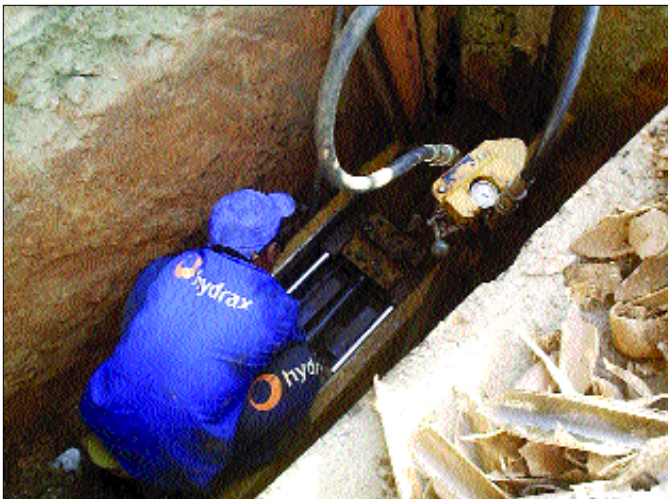
A Hammerhead HB3038 pipe bursting rig in operation on the City of Jaguariuna pipe replacement project.
